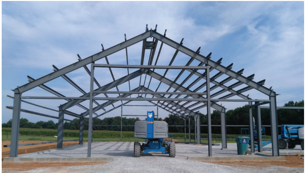
The outline of the future St. Francis of Assisi church is visible in this photo, which was taken on July 20, 2017. Since this picture was taken, vinyl has now been placed on the parish hall portion of the structure. Photo courtesy of St. Francis of Assisi Parish.
