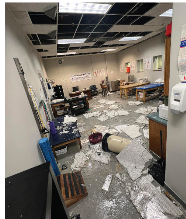
COURTESY OF BRESCIA UNIVERSITY Severe damage to Brescia University is seen in this photo taken after the hail that impacted western Kentucky in the early morning of March 15.
